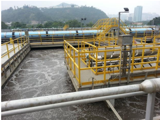
Sewage Treatment Works (污水处理厂)
